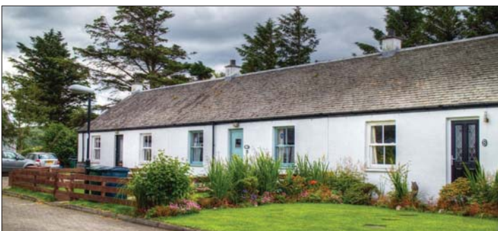
New, inappropriately small, chimneys
