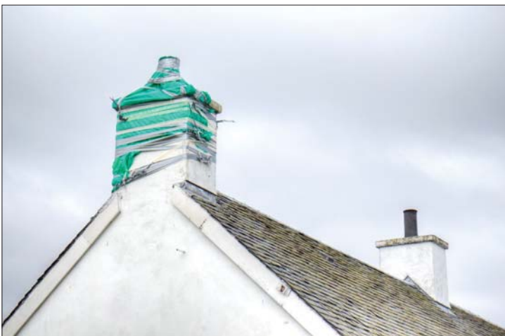
Chimney requiring maintenance
